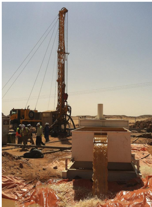
Airlifting after jetting: formation sand removed from the gravel pack by WellJet.
